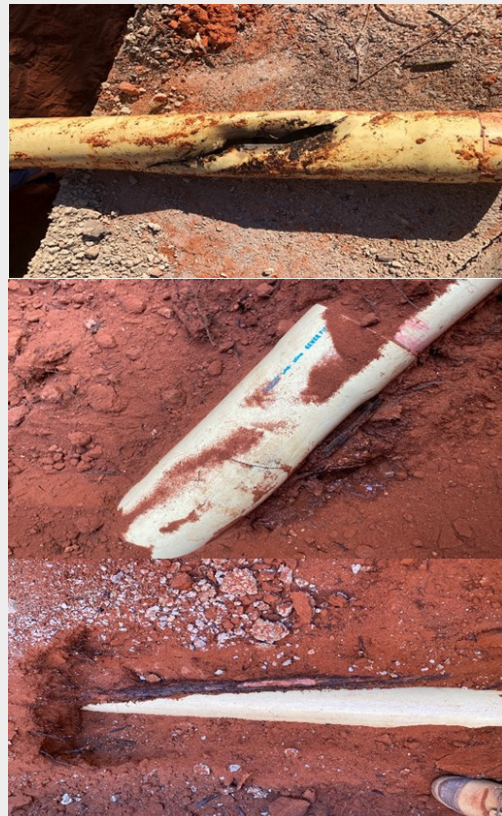
Tree root incursion in a section of sewer mains.
