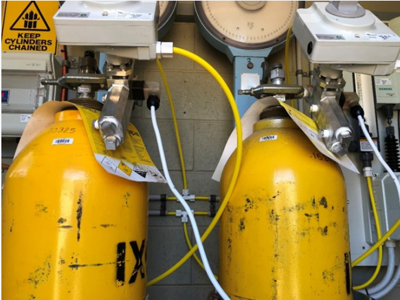
Drip legs on the chlorine dosing system.
