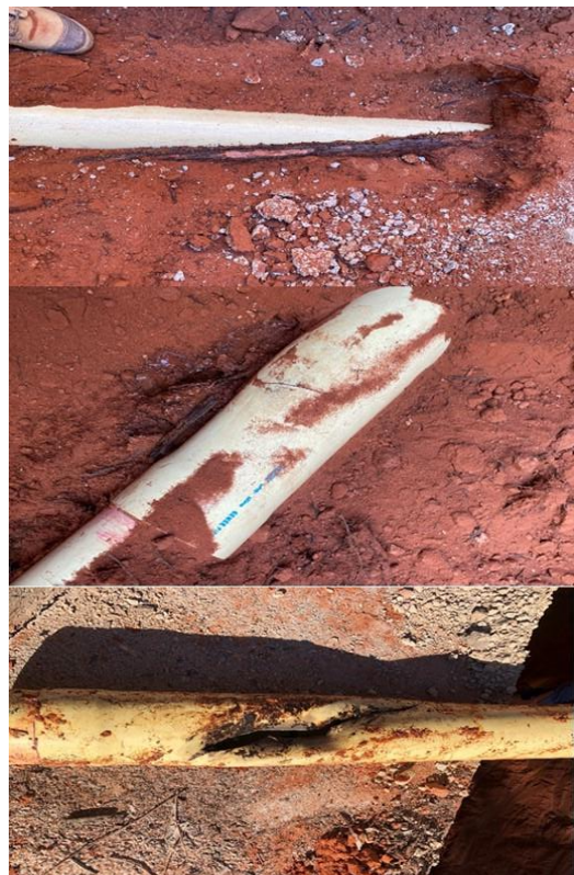
Tree root incursion in a section of sewer mains.
