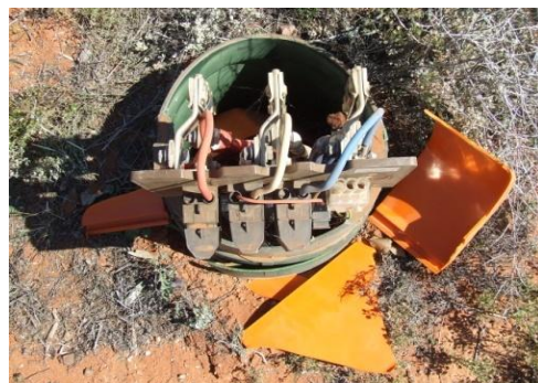
Section Pillar damaged by "off roading" Vehicles.
