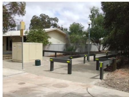
Stuart Rd walkway adjacent transformer S7 - fencing was upgraded for OHSW clearances and general beautification
