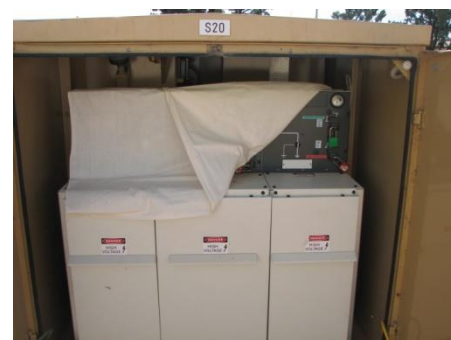
Due to high dust contamination, we have installed dust covers to help protect Ring Main Unit mechanisms
