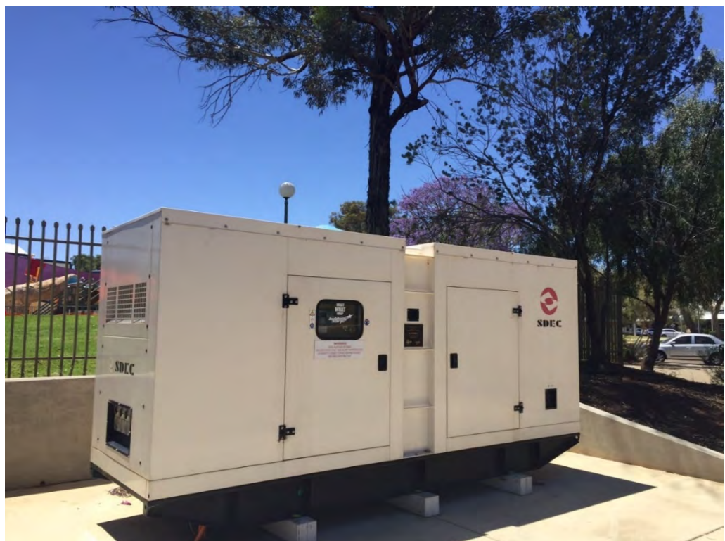
Roxbylink's diesel generator
