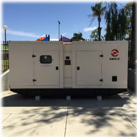
New generator for back-up power to roxbylink
