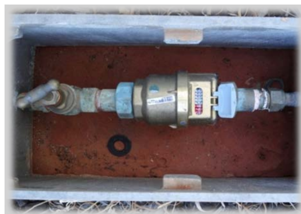
New 20mm water meter
