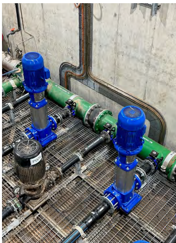
New Pumps at Town Water Supply (part of our pump replacement program)
