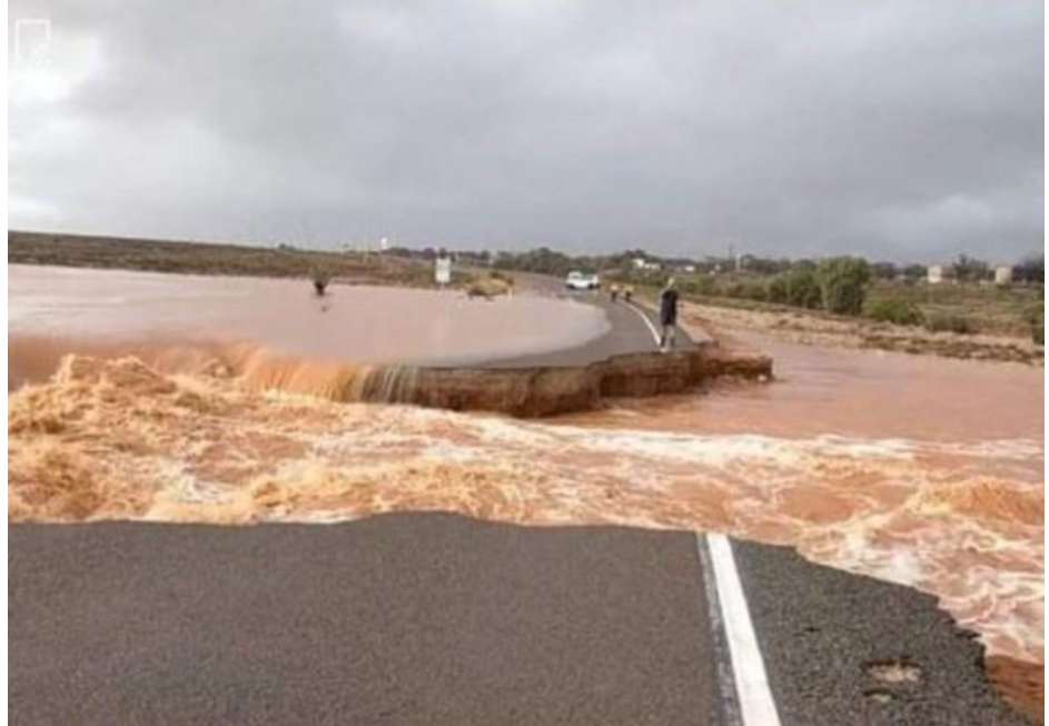
Flood waters washed away a large section of road between Woomera and Pimba in January 2022, cutting supplies to Roxby Downs and leaving some residents stranded.
