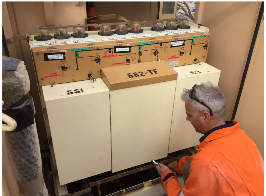
SA Power Networks maintaining a high voltage switch at the Roxby Downs Area School
