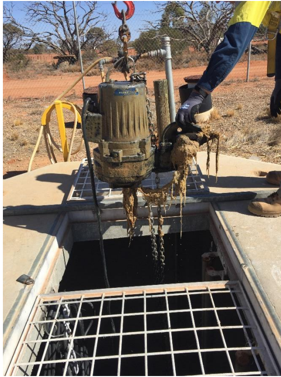
Pump at Station H requiring frequent maintenance
