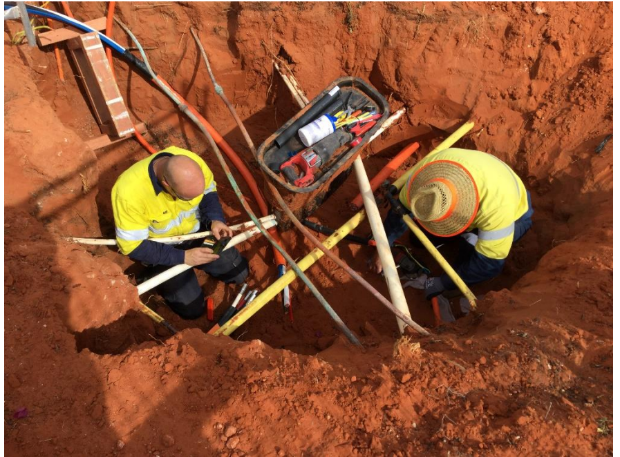
Cable repairs in a trench – Corner of Agonis Road and Maireana Circuit
