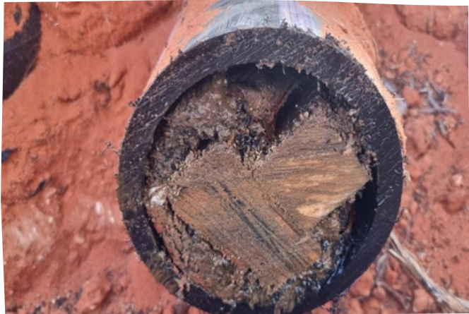
The pipe from the anaerobic weir to Primary Dam 3 was blocked at the elbow.
