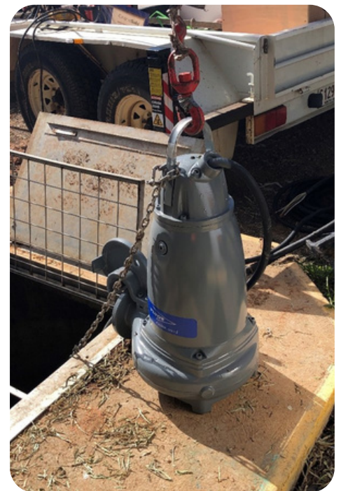
The new pump at Pump Station A being installed as part of the replacement program.
