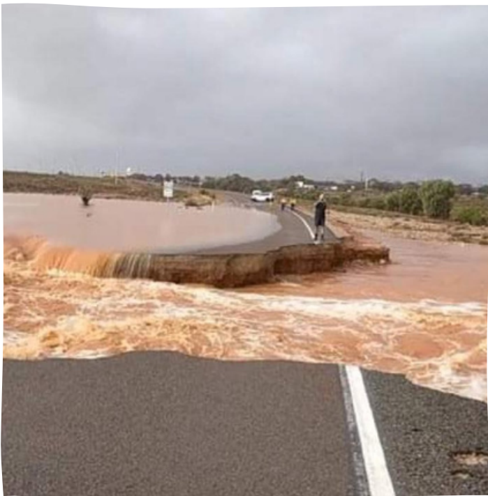
Floodwaters washed away a key section of road between Woomera and Pimba leaving residents stranded and disrupting supplies.
