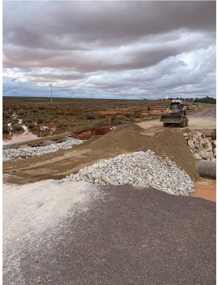
Contractors had to wait several days for the water to subside before the repair work could begin.
