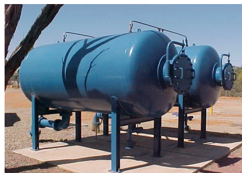
Hydro tanks at town water supply
