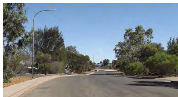
35 Watt LED lights installed in Quandong St. The conversion program will continue over 5 years
