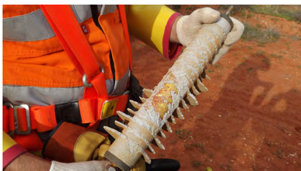
One of the 3 Surge Diverters damaged by birds
