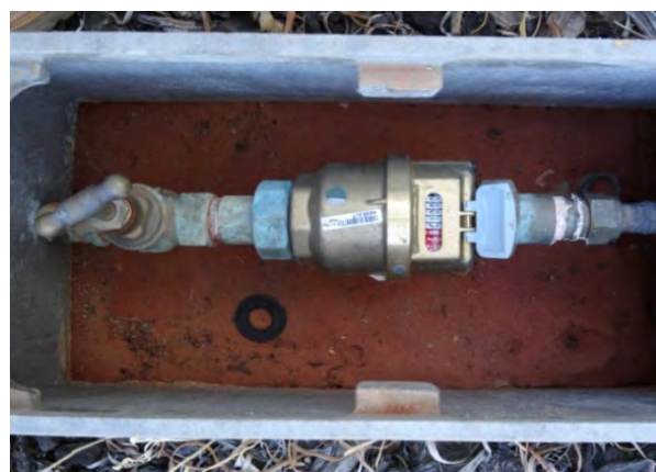
New 20mm water meter
