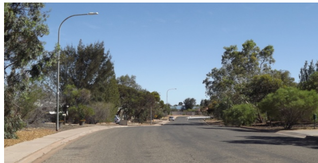
New LED light trial in Quandong St with 10 35W lights installed. The new Lights are also connected to a new Electronic Control system
