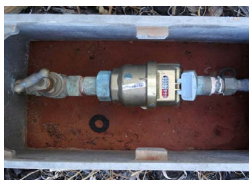
New 20mm water meter
