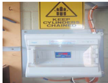
New chlorine gas detector at sewer lagoons treatment shed
