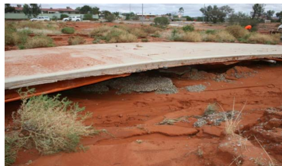
Some streets needed cleaning others needed shoulders repaired
