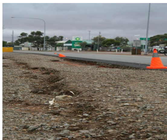
Road edges needed replacing in some areas of the township
