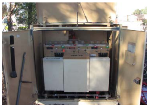
Old model RMU at Roxby Caravan Park Transformer before replacement
