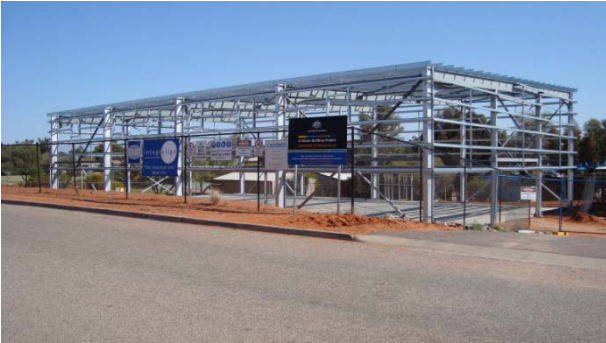
Building works at St Barbara's School – one of the few large scale development project in Roxby Downs
