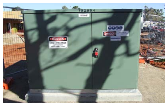
New SAPOL Transformer
