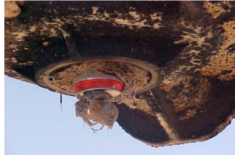
Pump Blockage by can in inlet. These blockages become very costly
