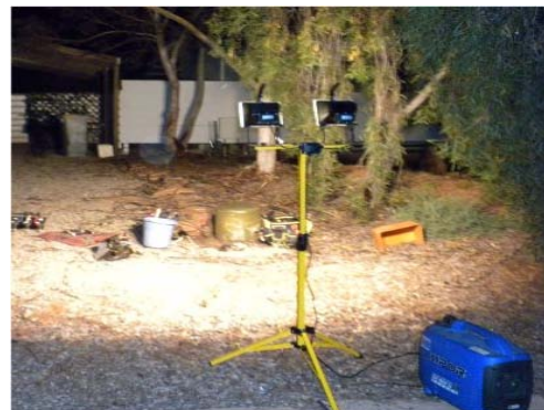
Midnight Repairs after a motor vehicle collided with a Section Pillar. A new pillar was needed - 2 Hours to repair.
