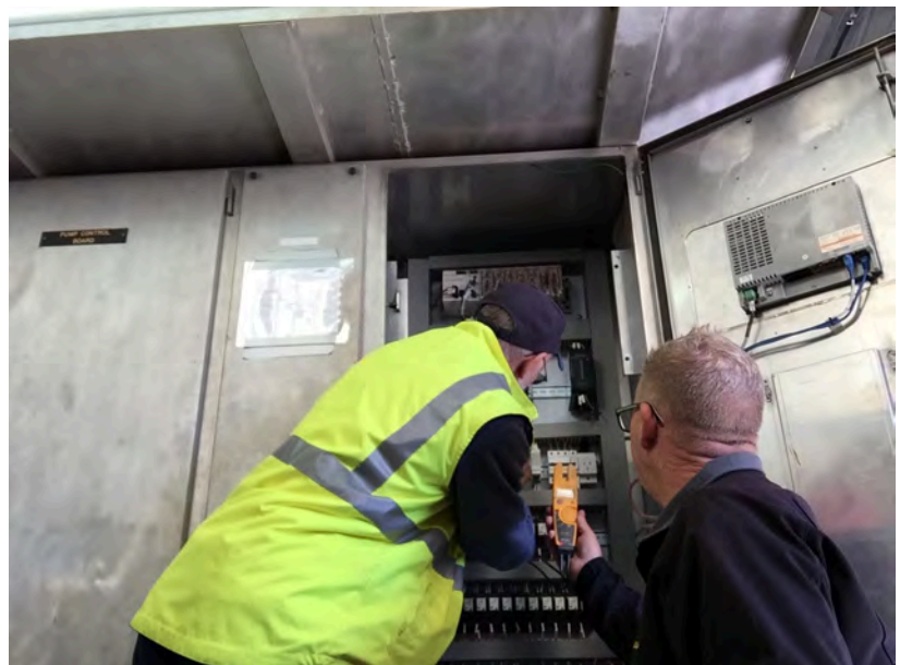
Works staff working quickly to rectify an issue that interrupted the power supply and water supply. The matter was quickly resolved within 15 minutes.
